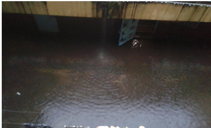
Figure 8: Photograph of one of the flooded residential flats in Ruiru town
