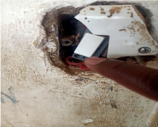
Plates 5.1: Electrical switch in a class
