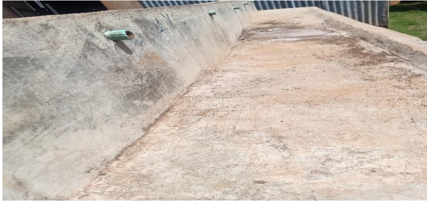
Plate 6.1: Showing an abandoned hand washing point in one of the schools in Nairobi County, Kenya.
