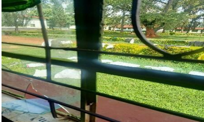
Plate 5.3: Showing a window with a grill and a broken glass in one of the in public secondary schools in Nairobi County, Kenya.
