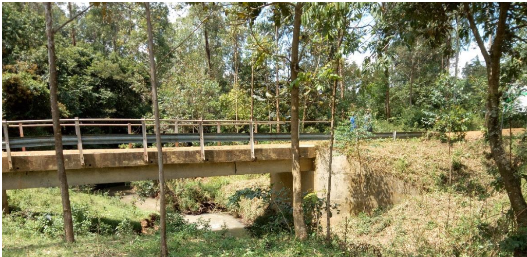
Plate 12: Ndombi Bridge with an access path passing by during the 2020 field visits
