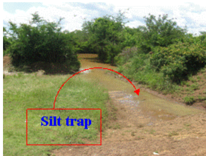
Plate 2 Water pan with failed silt-trap (in the lower RNB)
