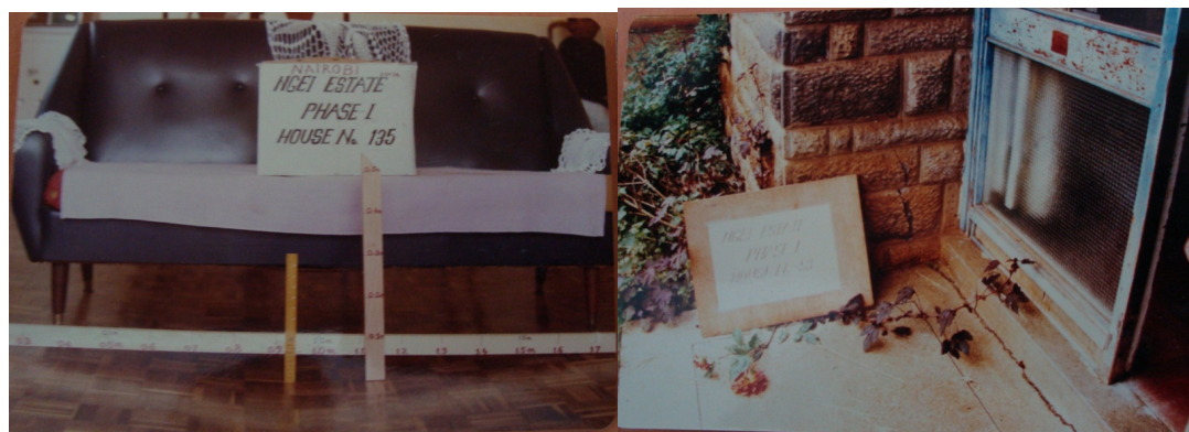
Figure 2: Distress in Ngei Houses (House No. 135 and House No. 53)
